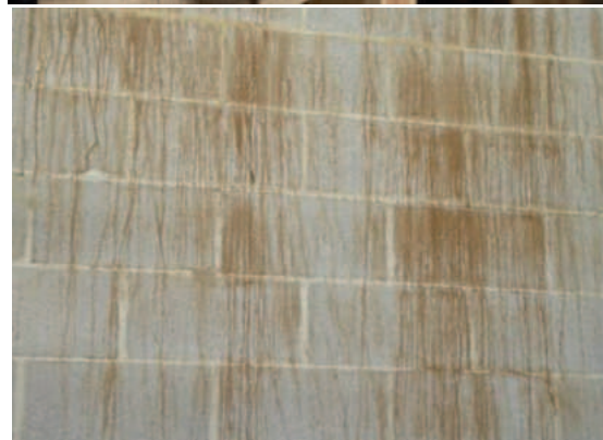
Above, tannins leaching out and staining oak panelling
